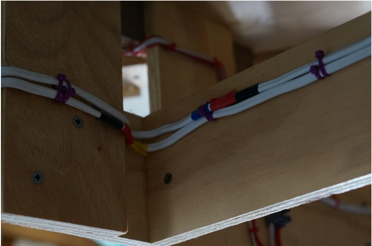
Or Stapled with Wire Ties sides/tops of the Sub Bases. All main Cables are secured together.
